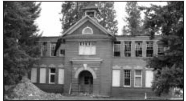
The old Clayton School building is undergoing a transformation. The old roof has been removed.
